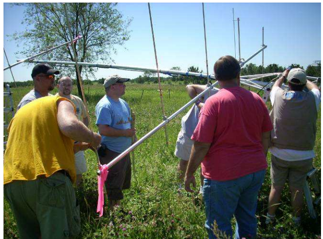
Fig 2. Plenty of help on the six meter array!
