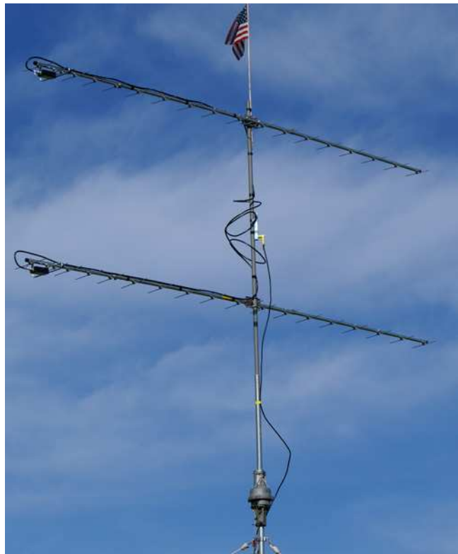
Fig 6. The 432 antenna stack.
